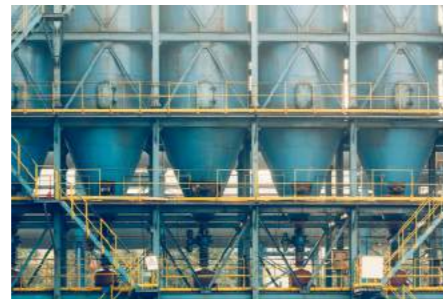
Gas transfer equipment on location
